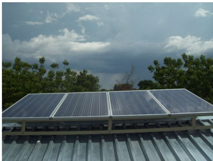
Photovoltaic system at the Okatale Combined School
